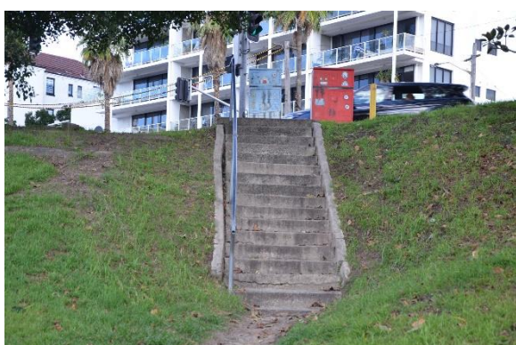
Figure 2.35 Mid twentieth-century concrete stair access in the southeast of the park. (Source: Ari Anderson, 2021)
