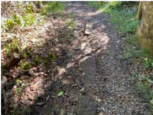
Figure 5: View of a portion of the unpaved pedestrian footpath with the attempts to fill the old tram route visible (Source: City Plan)
