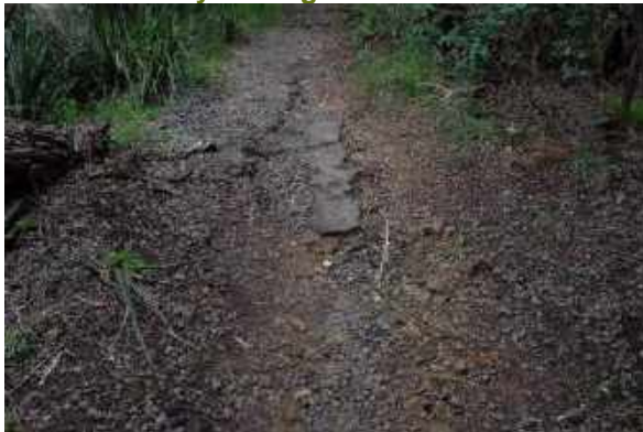
Figure 5-21. Example of a partially eroded bitumen footpath within the study area.
